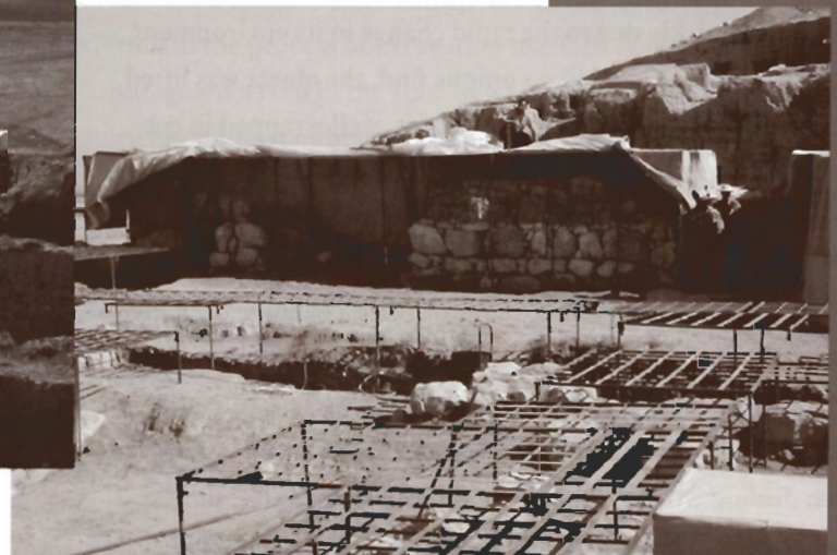
Left: A general view of the service wing of the Royal Palace, looking southwest. Tightly fitting canvas tents cover the metal cages to provide protection for the walls. Right: The covers can be quickly lifted to reveal the state of the walls. Photos: The International Institute for Mesopotamian Area Studies (images V13d8402 and V13d8567).
